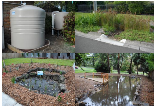
Examples of stormwater control measures installed as part of the research (clockwise from top left: residential rainwater harvesting tanks; roadside infiltration basin; large scale infiltration basin; and residential rain garden).
